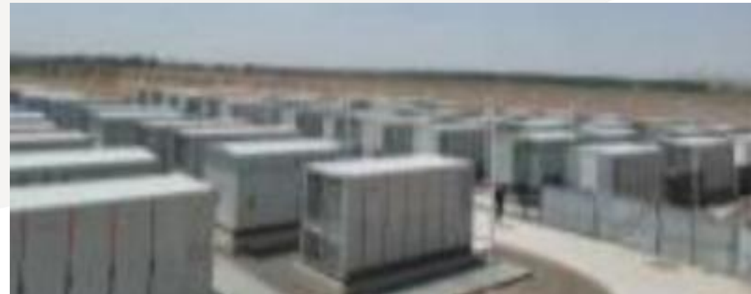
Belgium project 126MWh energy storage project
