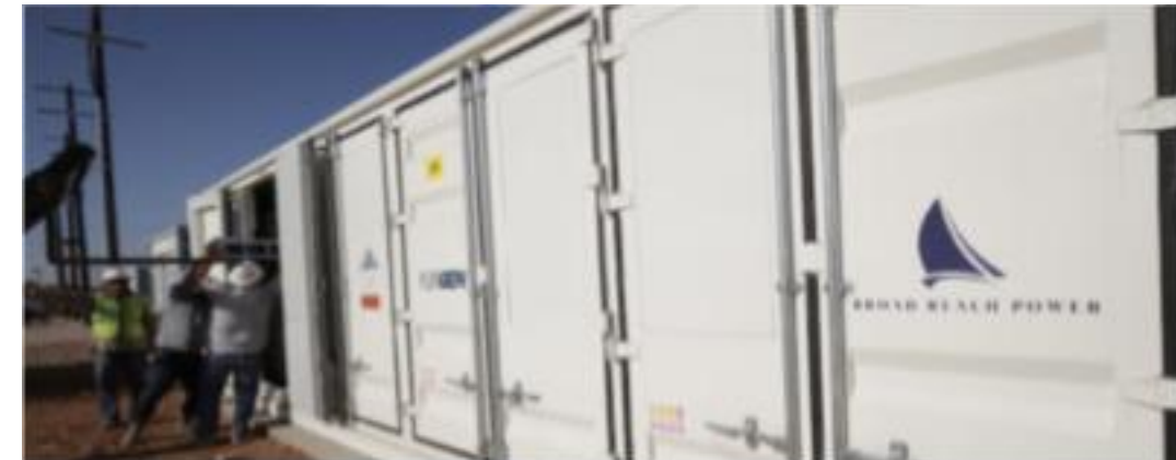
Cascade Energy Storage Project 117.5MWh California, USA
