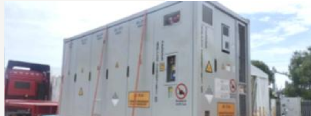
Bulgaria 7.45MWh photovoltaic distribution and storage
