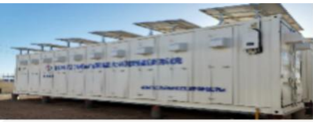
Guazhou, Gansu 12MWh Photovoltaic Energy Storage Project
