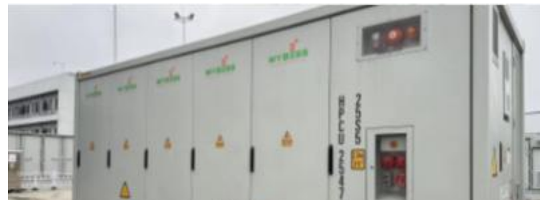
The 'MY BESS' project Malaysia sample 3.7 MWh
