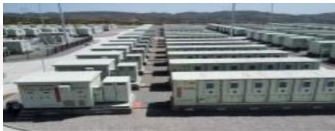
Ningxia Huarun Haiyuan 200MWh/400MWh
